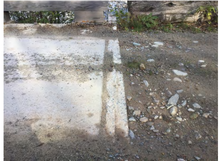
Left abutment ballast wall appears to have been cut
