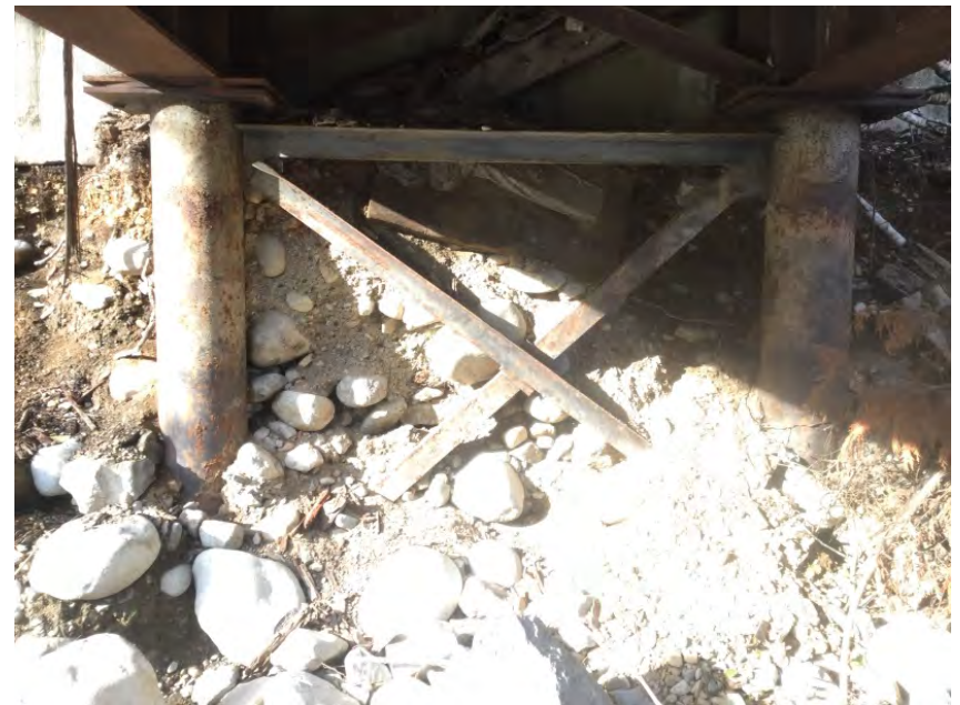
Over steepened fill behind right bank abutment
