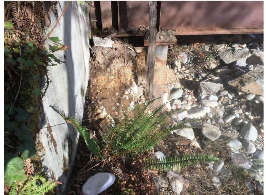
Over steepened fill behind ballast wall at right bank
